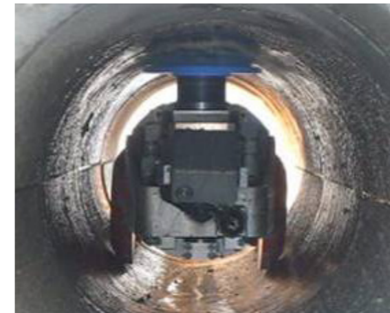
Roboter in Position
